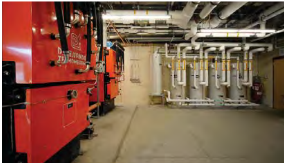
Wood Chip Boiler - Lebanon Middle School
